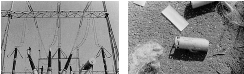
Figure 6. Left: Transformer and distributor installation of Nikola Tesla thermal electric power plant upon which cluster bombs with carbon fibers were thrown, causing short circuits and breakdown of the system, 2 May 1999. Right: Carbon fibre insert from a cluster bomb.
